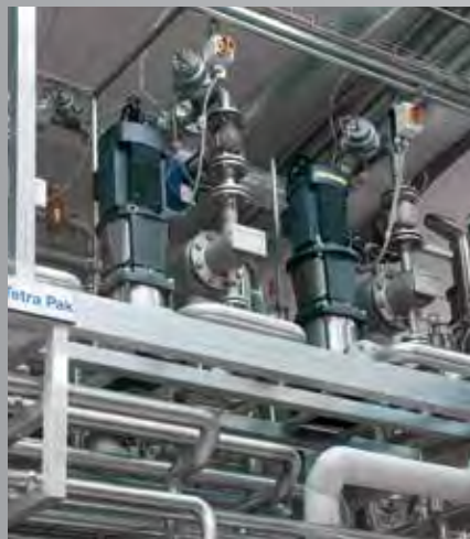
CR pumps installed in a dairy plant
