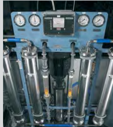
CRN 5 installed in a water treatment plant
